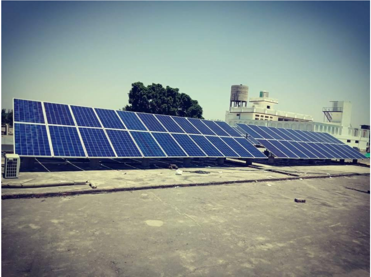
50KWp Solar Grid Tied Power Plant at Gurudwara Nanaksar Sahib, Jagraon
