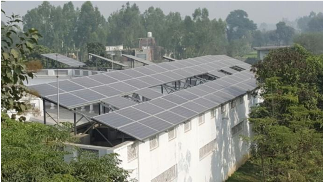
55KWp Solar Grid Tied Power Plant at Hari Singh Public School, Chella
