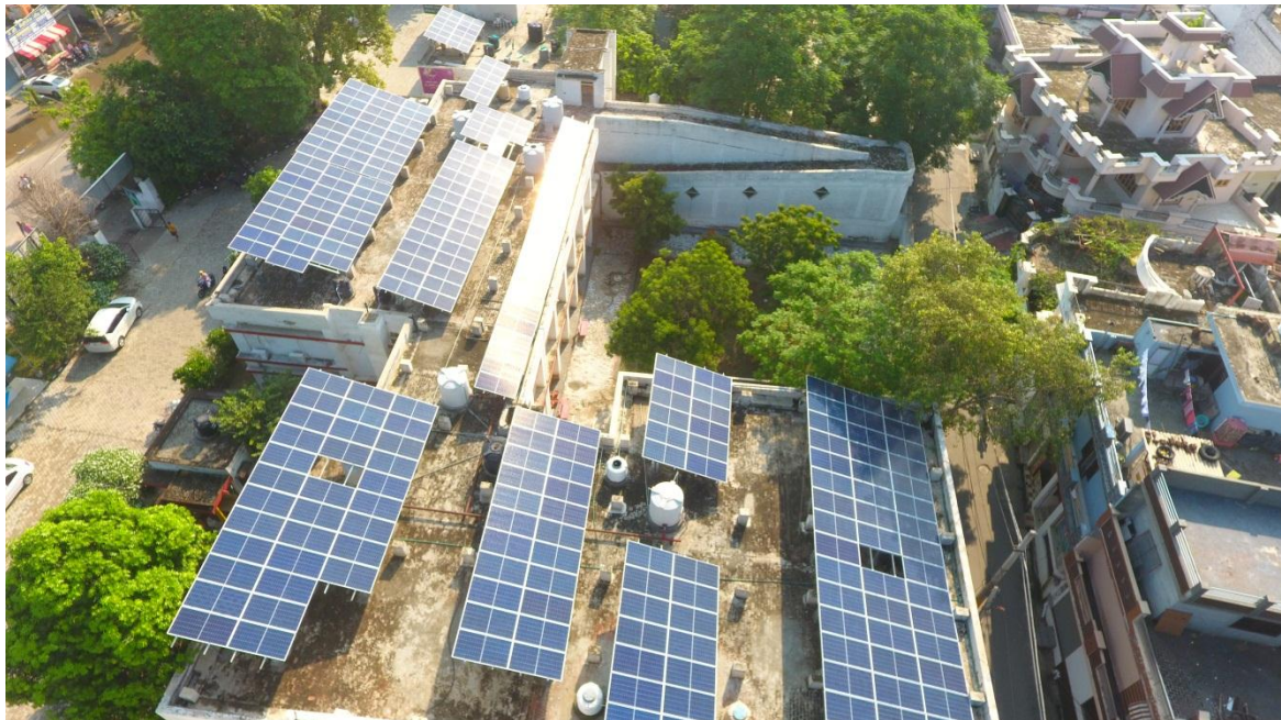
150KWp Solar Grid Tied Power Plant at Civil Hospital, Sultanpur Lodhi ( Under Smart City Sultanpur Lodhi Project )
