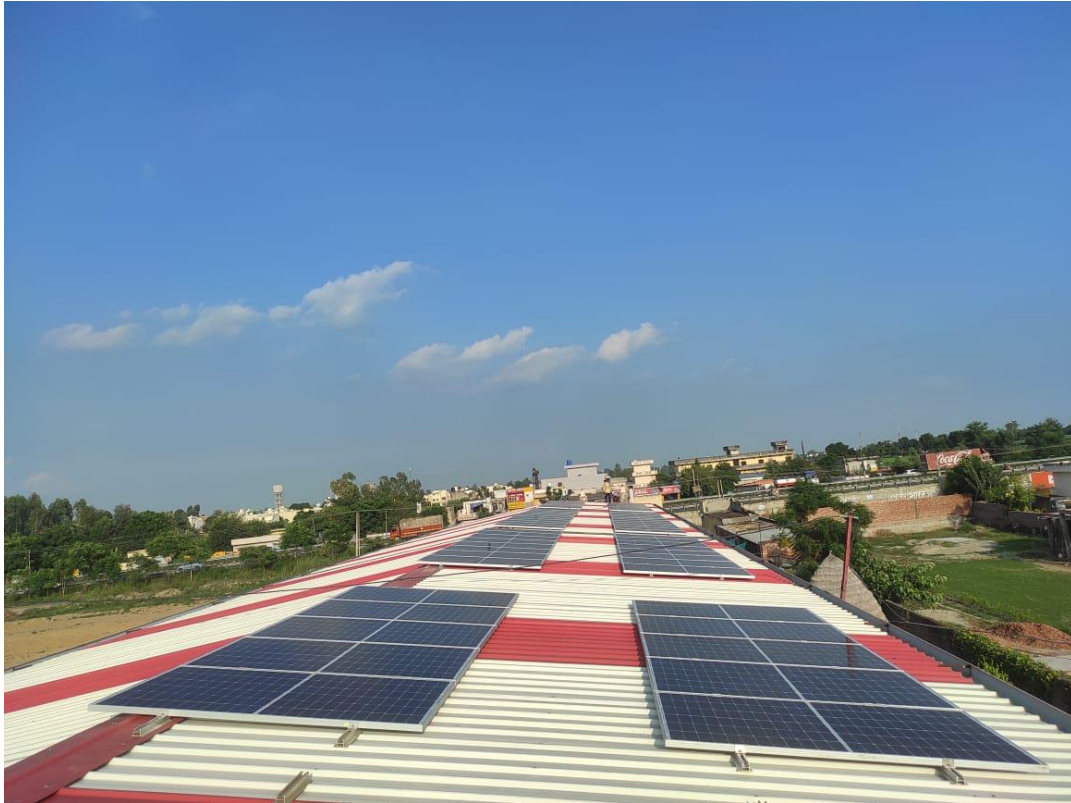
50KWp Solar Grid Tied Power Plant at Prabhakar Marbles, Phagwara
