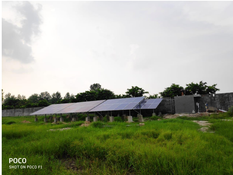
30KWp Solar Grid Tied Power Plant at GNA Aviation Wing, Phagwara
