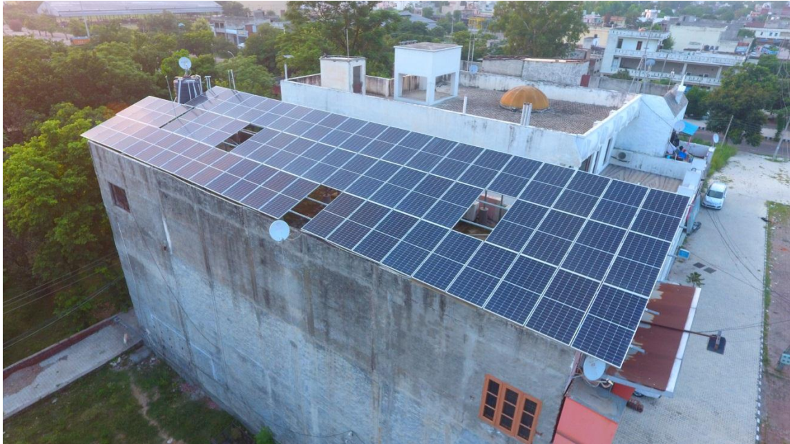
30KWp Solar Grid Tied Power Plant at JD Restaurant, Hoshiarpur
