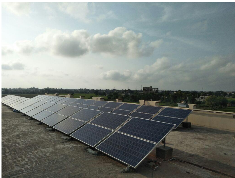
20KWp Solar Grid Tied Power Plant at NBSD School, Sangrur
