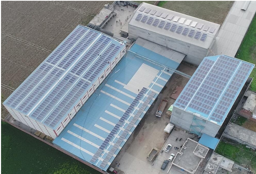
380KWp Solar Grid Tied Power Plant at Guru Nanak Cold Store
