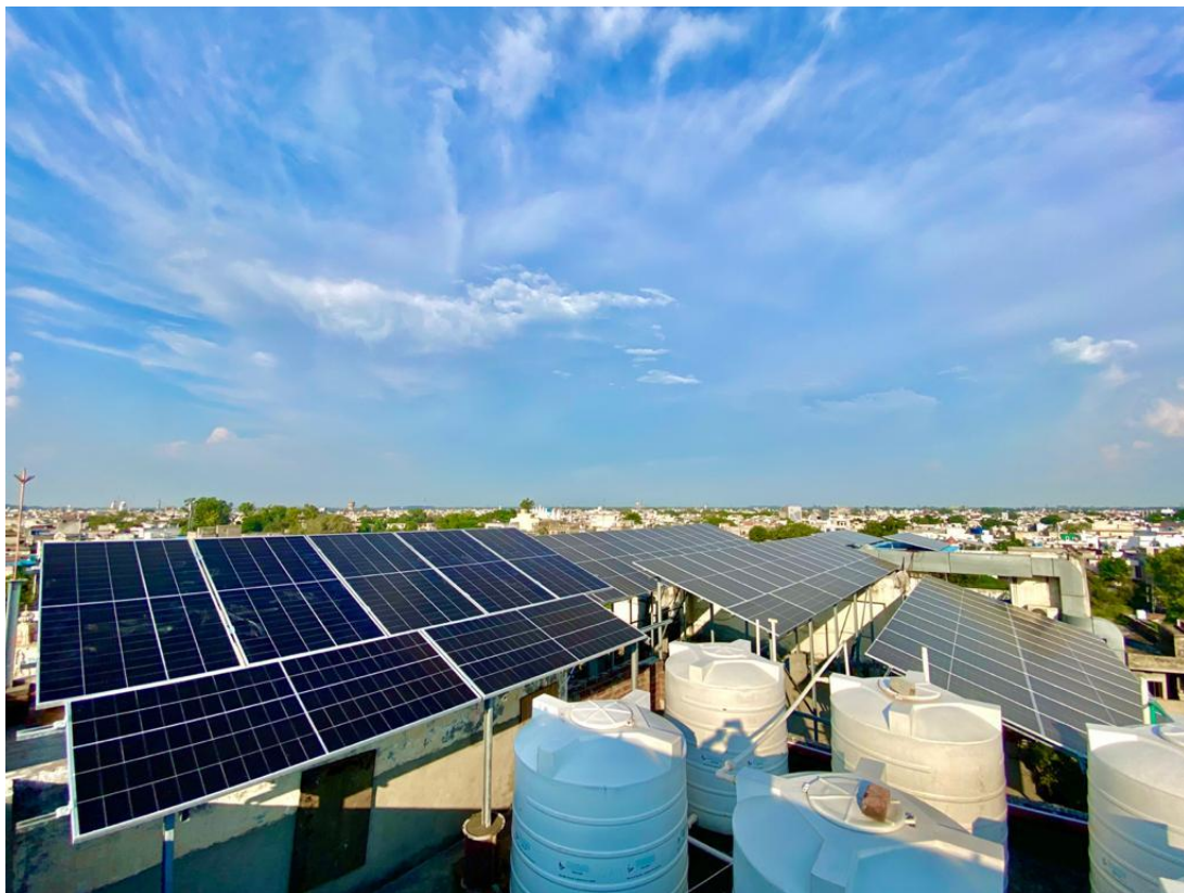
70KWp Solar Grid Tied Power Plant at Poonam Hotel, Phagwara
