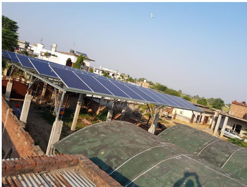
20KWp Solar Grid Tied Power Plant at Khehra Finance, Sarchur
